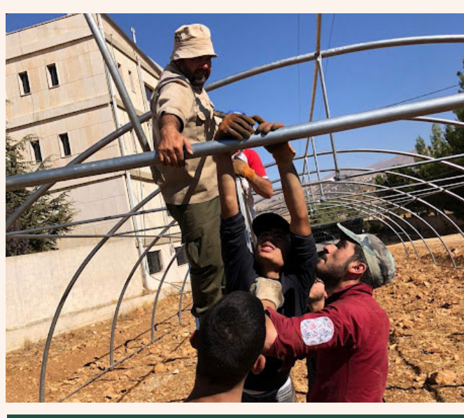
The team installs a greenhouse at the Technical and Vocational Education & Training (TVET) school in Rachaya
